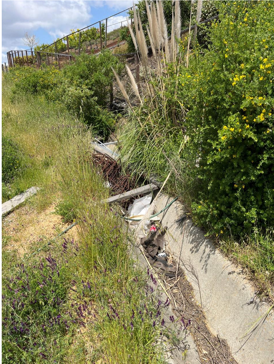
Trash and construction debris accumulated in concrete-lined ditch.
