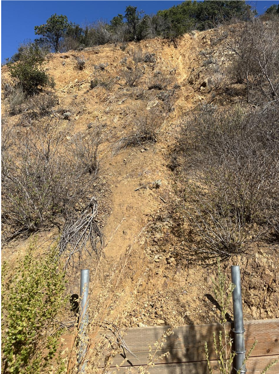
Erosion gully formed above drainage ditch and wood-lagging debris wall, eroded material deposited behind wall and in drainage ditch. From previous walk fall 2022 since access to this area was blocked.
