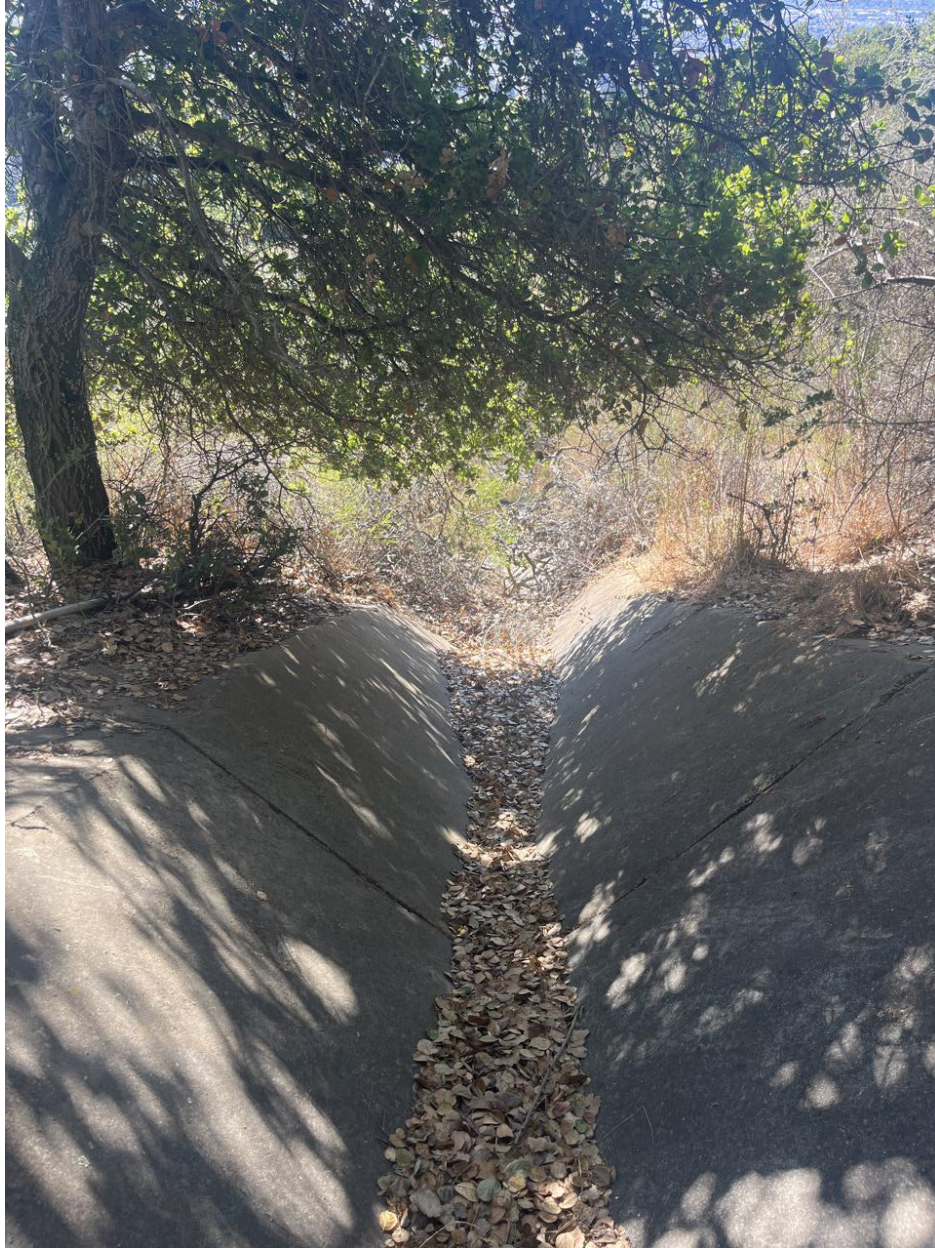
Site Condition A – Tree debris blocking concrete-lined drainage ditch.
